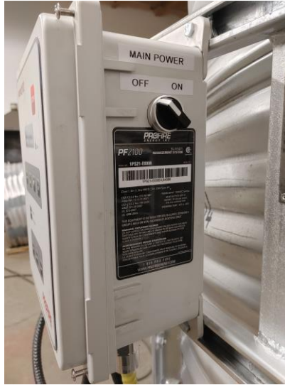
Figure 4 – Profire Main Power ON/OFF Switch Location
